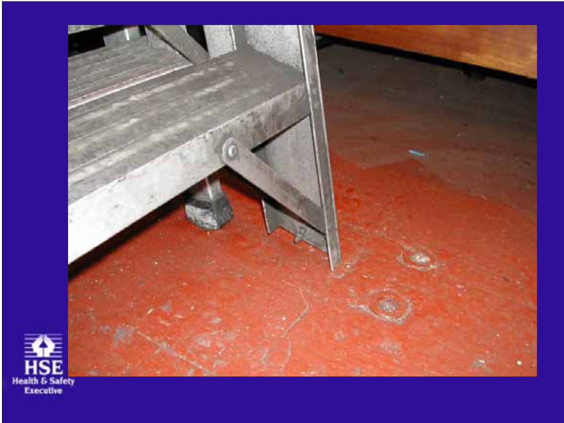
Missing foot, will lead to wobble and reduced slip resistance – Could be repaired
